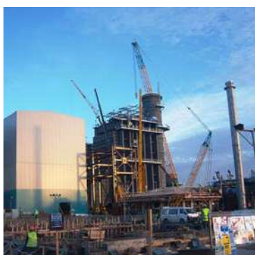
DENIZLI 775MW COMBINED CYCLE POWER PLANT
