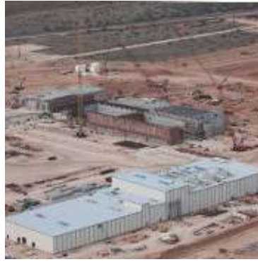
LES NEF NATIONAL URANIUM ENRICHMENT PLANT
