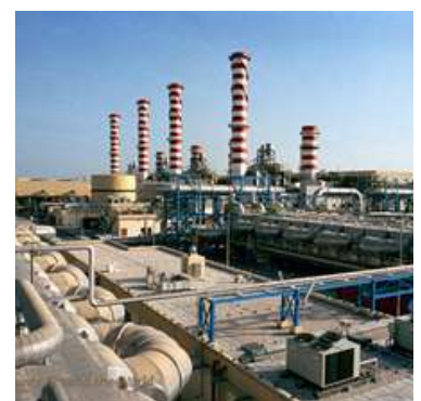
RASLAFFAN, EPIC SUPPLY OF SEA WATER TO LNG1, QP BY CCIC - TECHNIP
