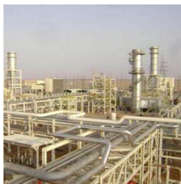
DODSAL & VEOLIA WATER STI, QARN ALAM STEAM PROJECT - PDO
