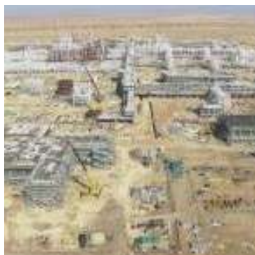
YIBAL KHUFF INTEGRATED OIL & SOUR GAS FACILITIES PROJECT, BY PETROFAC
