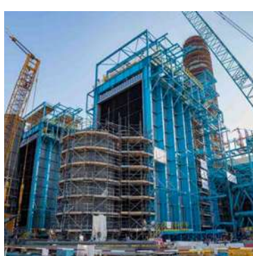
AL LAYYAH COMBINED CYCLE POWER PLANT, SEWA
