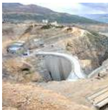
ALSTOM AUSTRIA GMBH, ERMENEK HYDROELECTRICAL POWER PLANT
