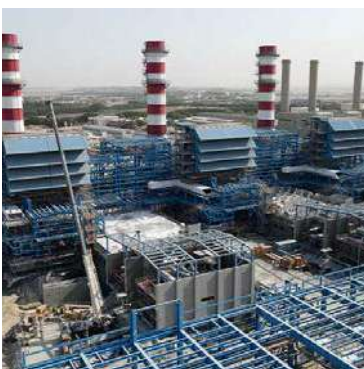
AL AWEER COMBINED CYCLE POWER PLANT, DEWA
