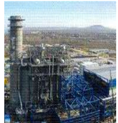
ANSALDO GEBZE COMBINED CYCLE POWER PLANT
